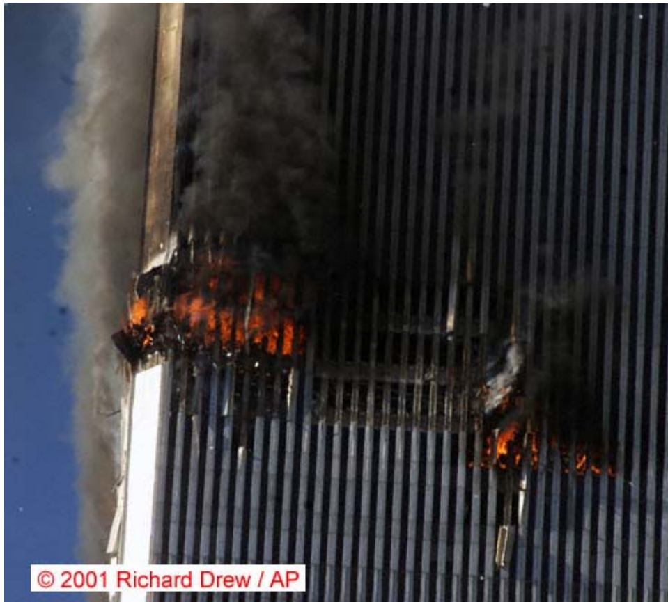
Figure 7–74. Impact damage to the northeast corner of the exterior wall of WTC 2.
