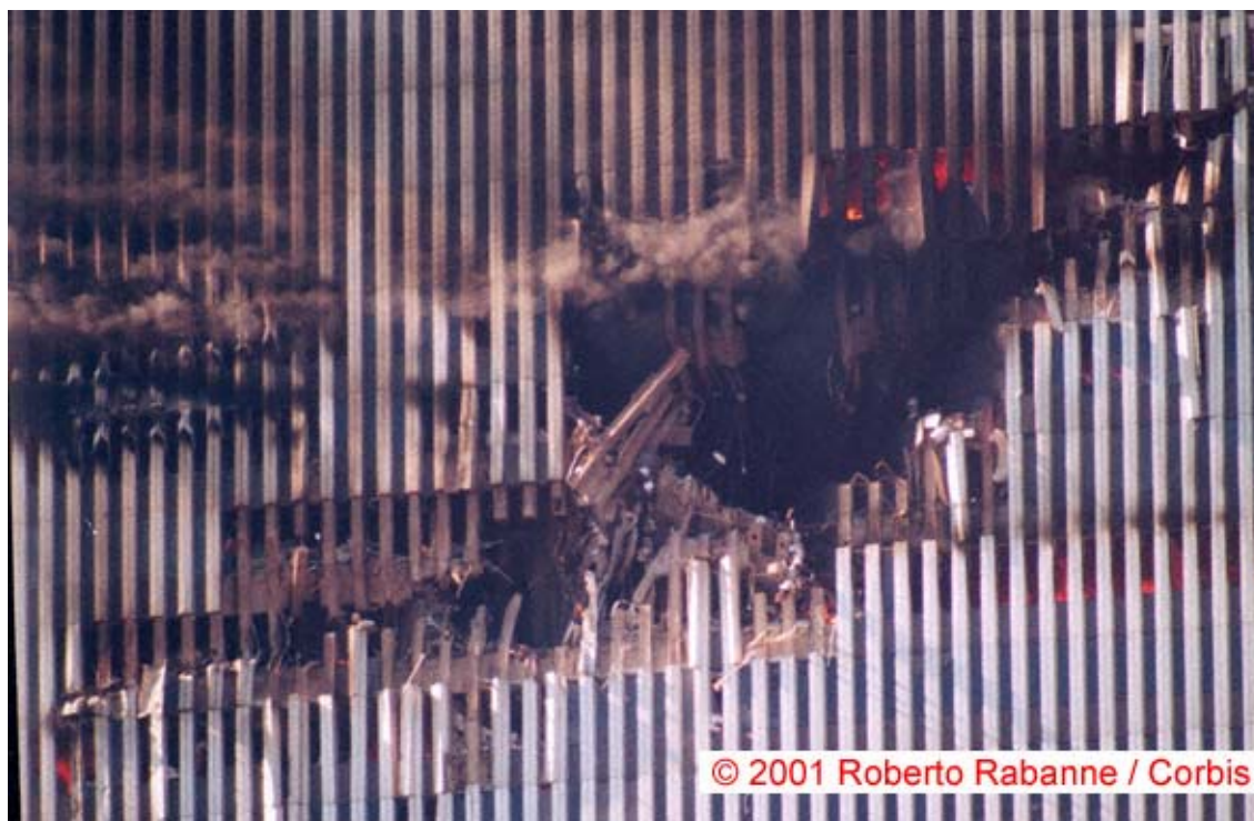
(a) Observed Damage
