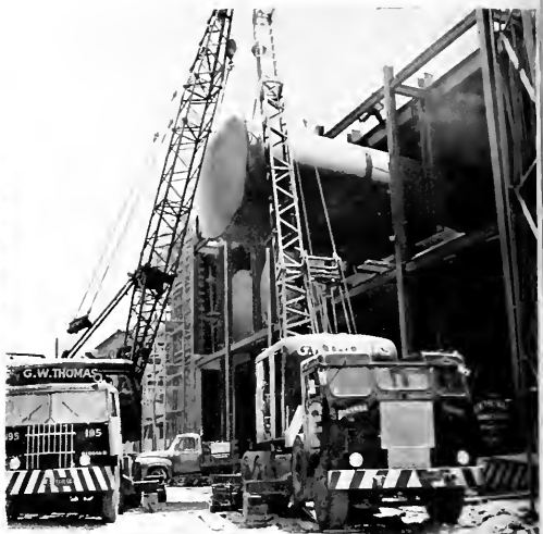
Today huge multi-wheeled diesel trucks and cranes manned by the same type of personnel carry on the tradition of the company.
