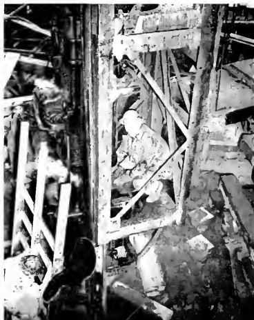
The finish of the pile-driving operation for the American Trust's new headquarter's building.
