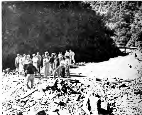
Members of the 1958 Grand Jury inspect site of new powerhouse
