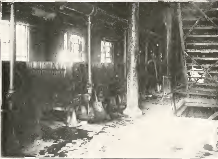
PRESSURE FILTERS, WHICH REMOVE ALL THE PURIFYING AGENTS
